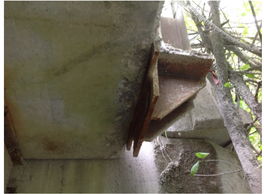
minor damage to upstream right approach deck panel under rail post
